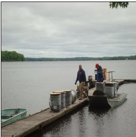
Figure 3. LFA System Installation, 2012 Photo courtesy of Cathy Freebairn
