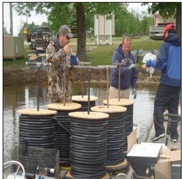
Figure 4. LFA System Installation, 2012 Photo courtesy of Cathy Freebairn
